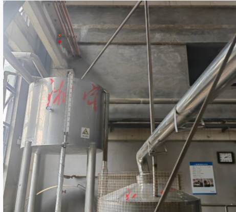
Sauce-Flavor Baijiu Workshop Cooling Water Reuse for Bathing Facilities
