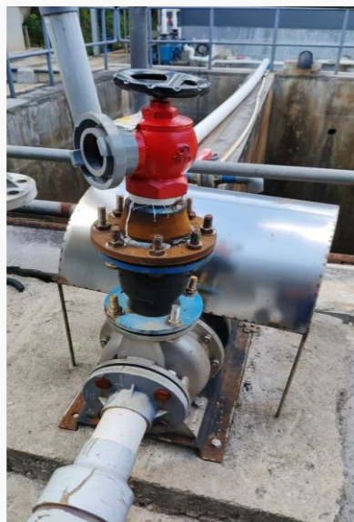
Wastewater Treatment Station Reclaimed Water Utilization for Landscaping Irrigation
