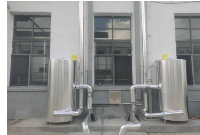
Heat Recovery System at Lidu
