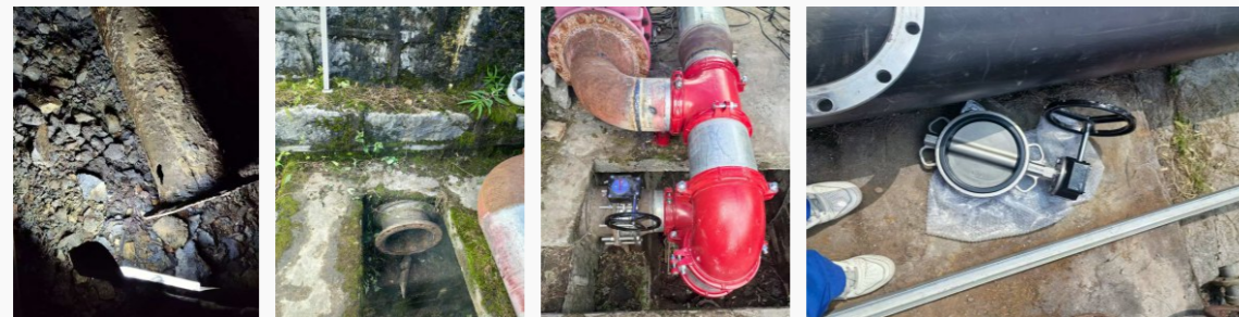
Modification of Pipelines and Valves in the Elevated Water Tank of the Shizipu Plant Area
