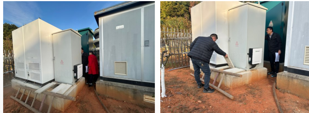
Lidu Distillery Routine Electricity Inspection
