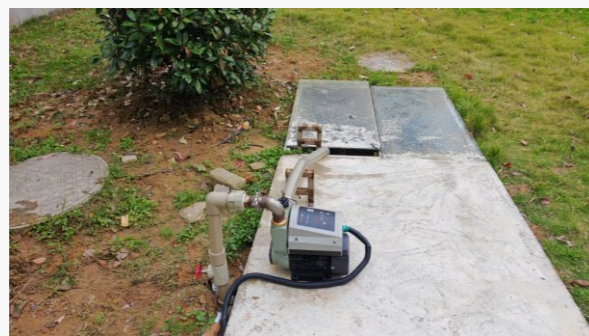
Zhaojiagou Plant Reclaimed Water Reuse Project
