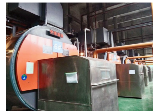
Natural gas boilers
