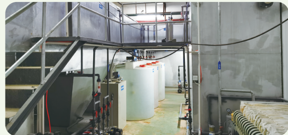
Self-built Wastewater Treatment Facilities
