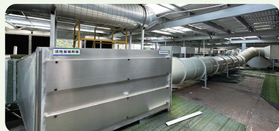
Waste Gas Treatment Equipment
