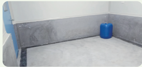
Medical Waste Liquid Temporary Storage Room
