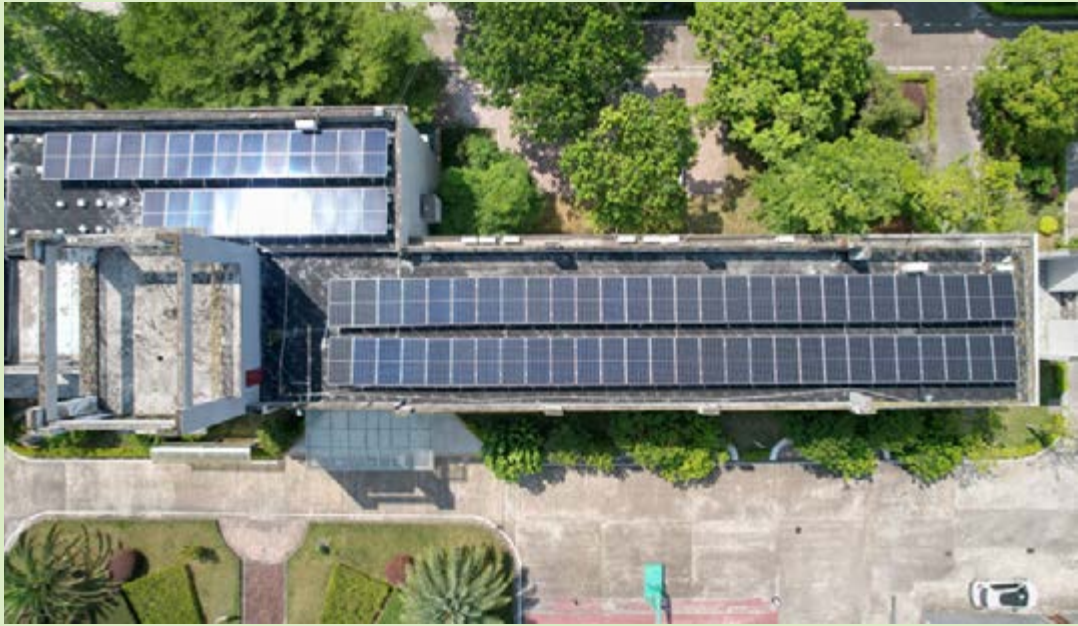
Distributed Photovoltaic Power Generation Project of Cangyu Company
