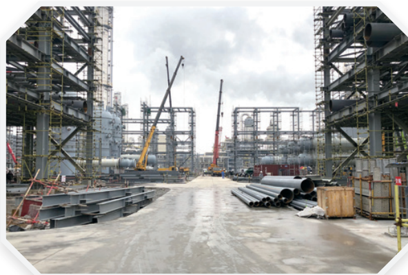
The ethylene project for Zhejiang Petrochemical won a number of awards for quality and construction management
