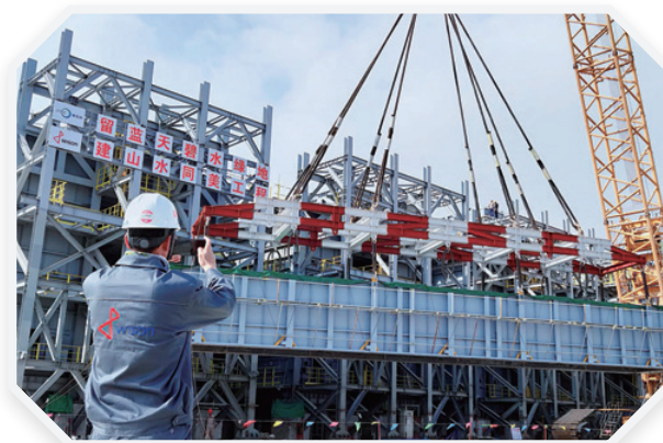
Wiscon Engineering has allocated more resources for construction staff, machinery and equipment in key projects since March
