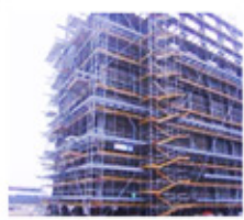
Operation above ground
