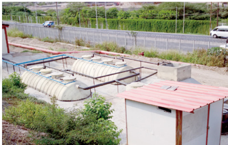
Sewage Recycling Treatment System
