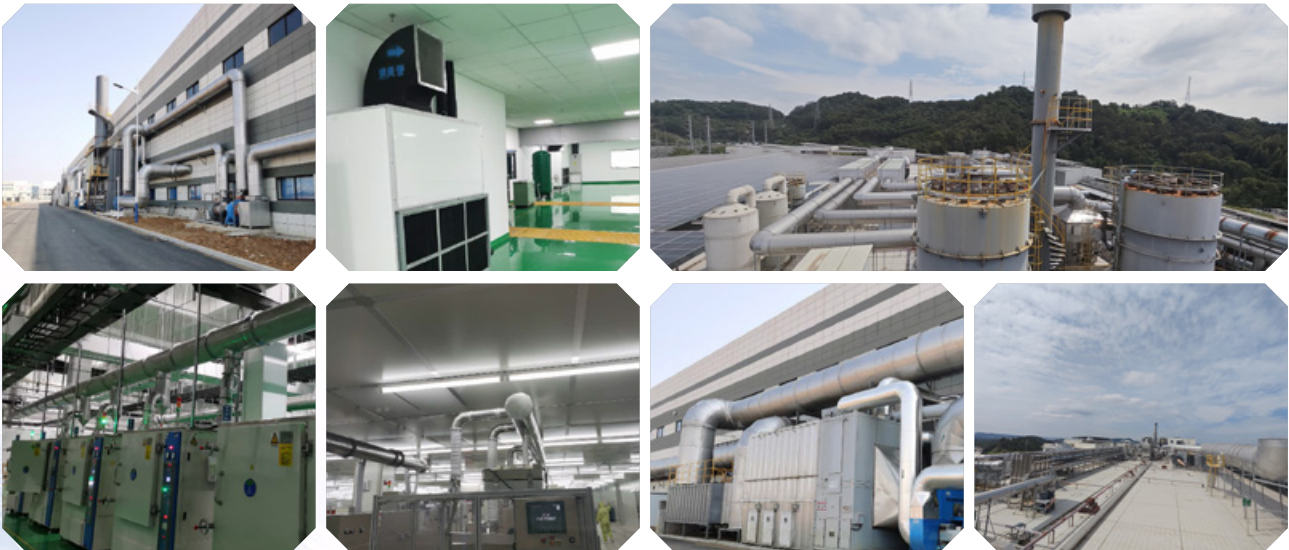
Exhaust Air Treatment Facilities 廢氣處理設施
