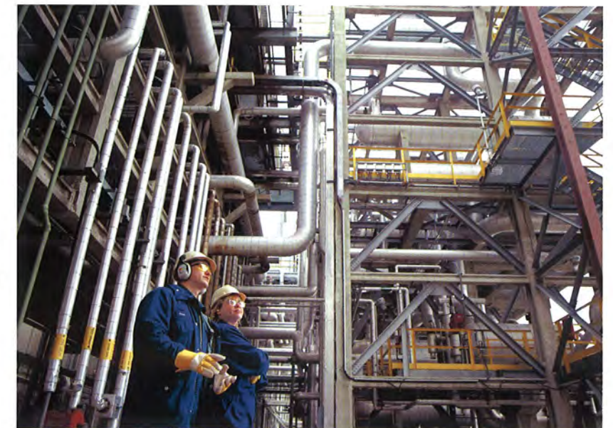
Husky Oil's heavy oil upgrader in Lloydminster, Saskatchewan, achieved record processing volumes of synthetic crude oil in 1999.
