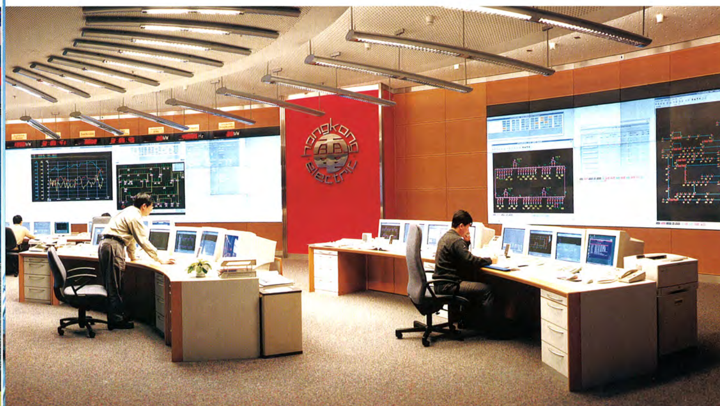
Hongkong Electric's new control centre acts as the nerve centre of the electricity supply system.
