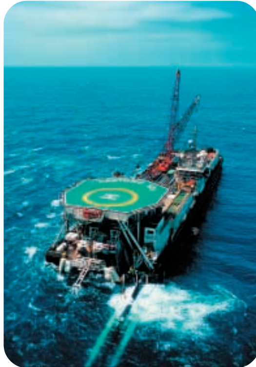
● A barge lays the new pipeline for Hongkong Electric to carry environmentally friendly natural gas from Shenzhen to East Lamma Island for future LNG-powered turbines.
