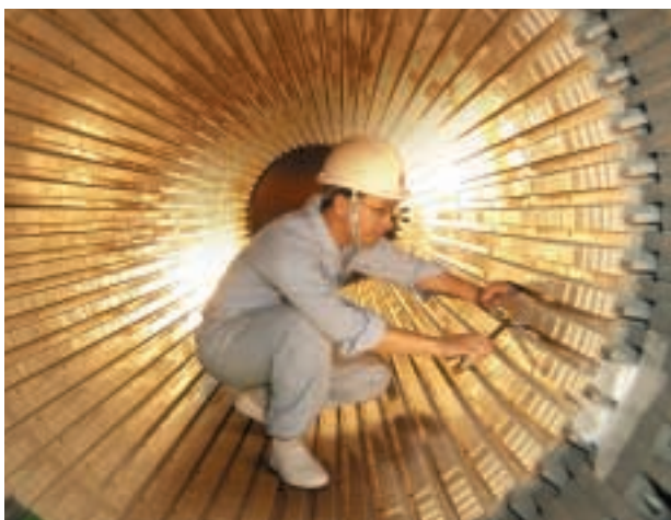
■ A technician carries out a regular inspection of a turbine generator as part of Hongkong Electric's continuous, preventive maintenance schedule. This constant attention to detail underpins the company's impressive record of 99.999% supply reliability.
