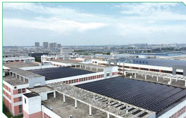
■ The rooftop solar energy facilities at the Everbright Sucheng Development Zone commenced grid-connected power generation in October 2024. It has a designed installed capacity of 40 MW, making it the Group's largest solar energy project by installed capacity.
