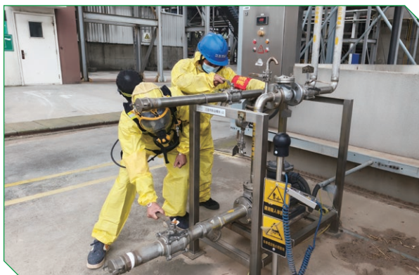
Emergency drill for ammonia leak at Shayang Integrated Biomass and Waste-to-Energy Project
