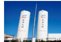
Industrial Gas Cryogenic Tank
