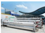
Hydrogen Storage Cascade for Stations
