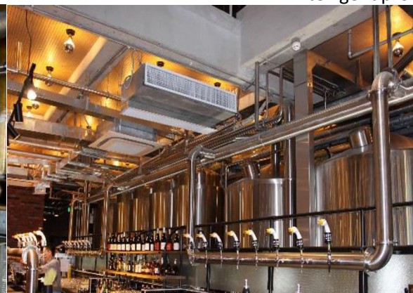
Craft beer technology, equipment, system and engineering
