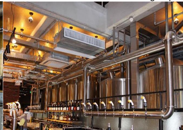
Craft beer technology, equipment, system and engineering
