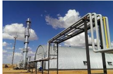
Wellhead gas recovery package
