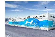
Skid-mounted hydrogen refuelling station
