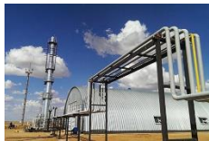
Wellhead gas recovery package
