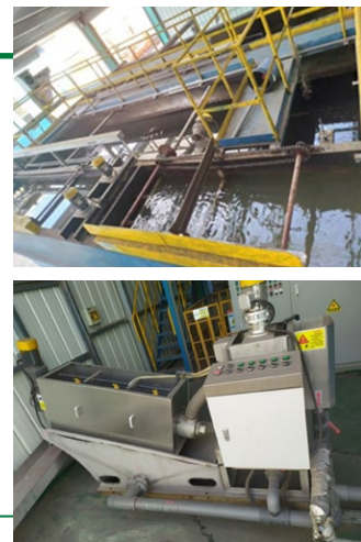
Water Treatment System of CIMC Sanctum
