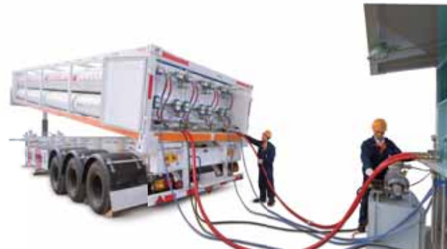
CNG refueling station system
