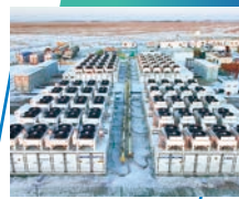
Distributed low-carbon energy stations
