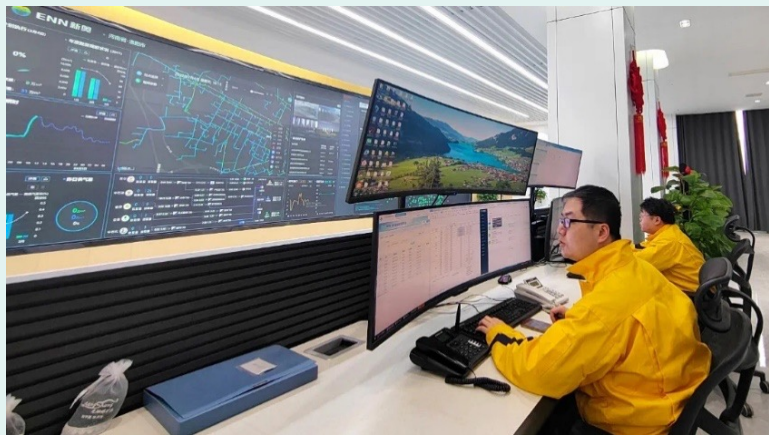
Smart Operation Centre
