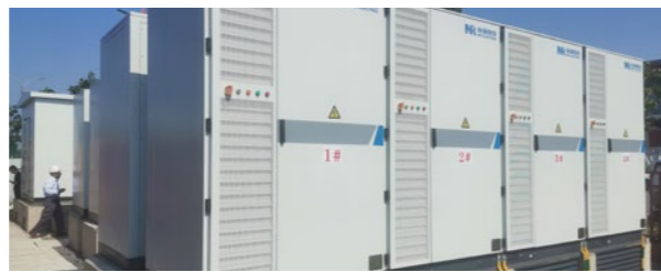
Energy Storage Project
