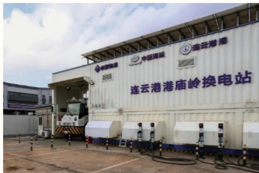
Battery-swap station at Lianyungang New Oriental Terminal
