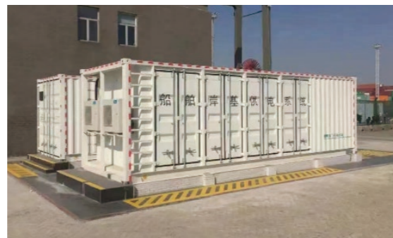
Vessel shore power supply system
