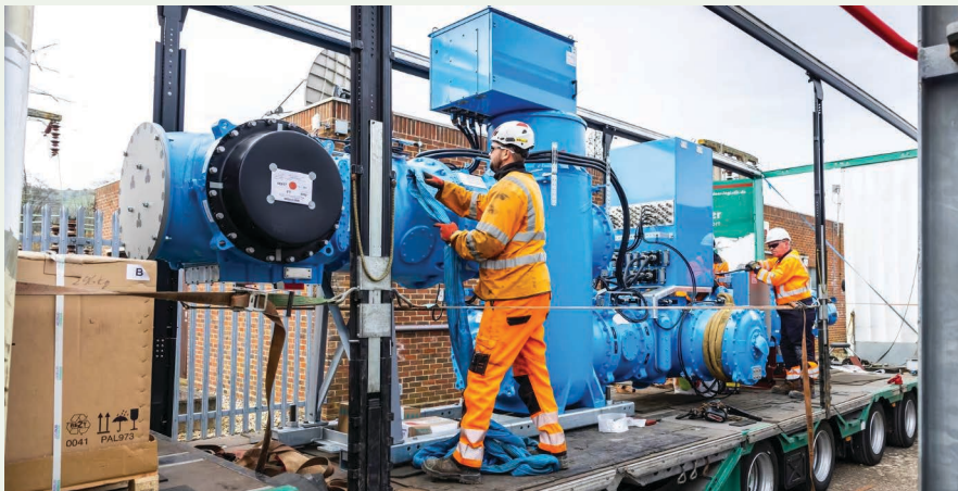
"Clean air" Gas Insulated Switchgear system at UK Power Networks.
