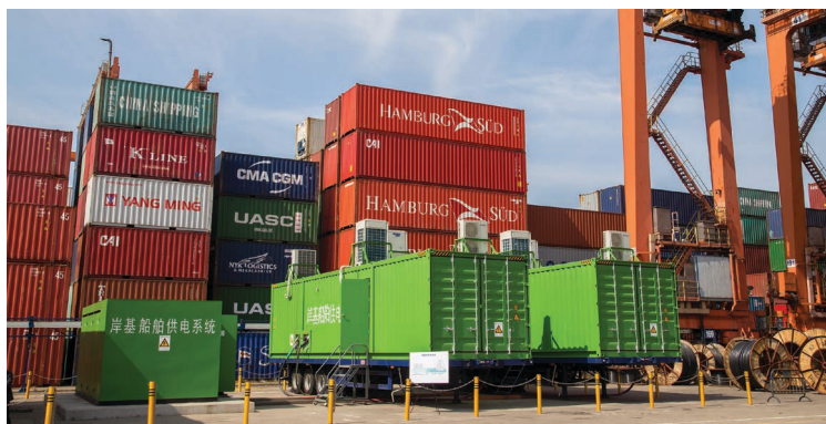
Shore power system at Hutchison Ports Yantian
