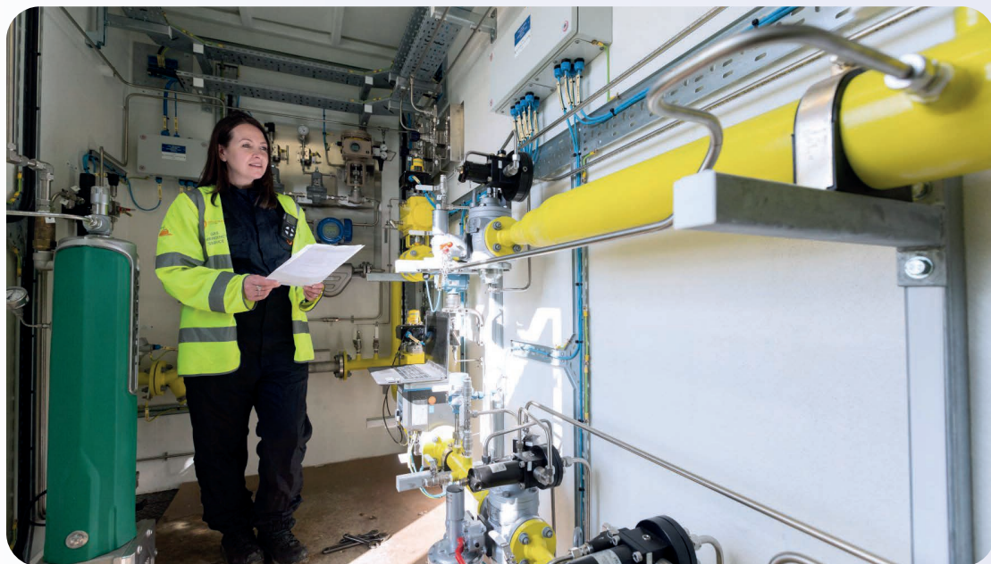
Wales & West Utilities 智能壓力控制系統
