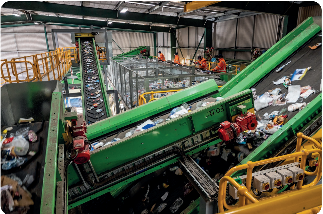
Resource recovery facilities, Enviro NZ
