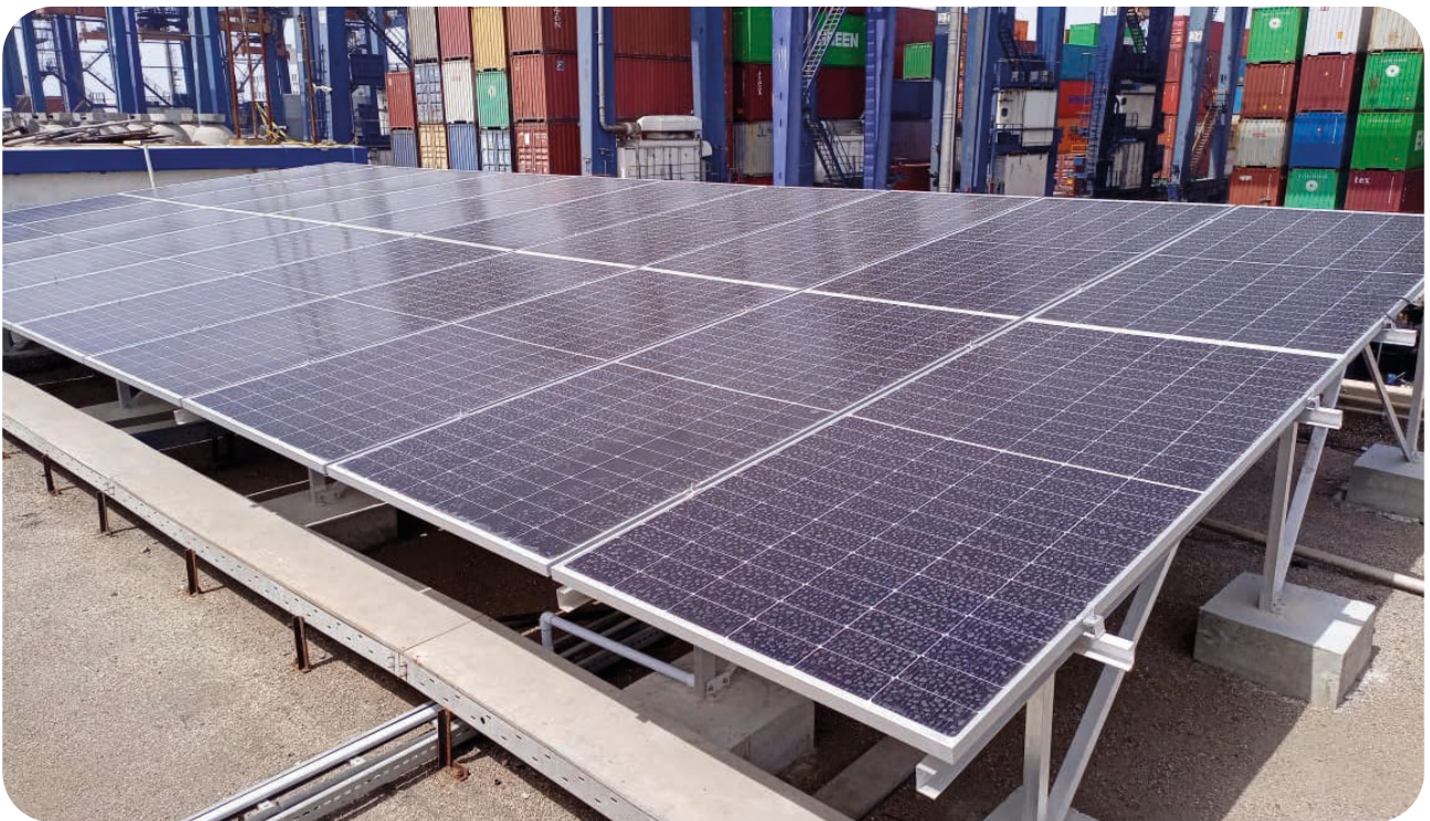
On-site solar panels, Hutchison Ports KICT
