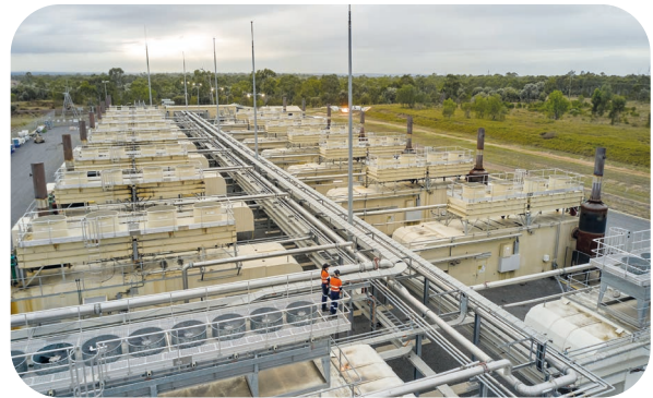
Waste coal mine gas powered stations, EDL
