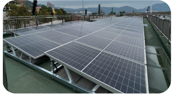
Solar panels at "A Square" Transitional House, HK Electric
