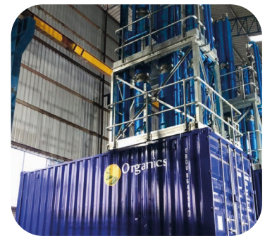
Ammonia capture from wastewater, Northumbrian Water
