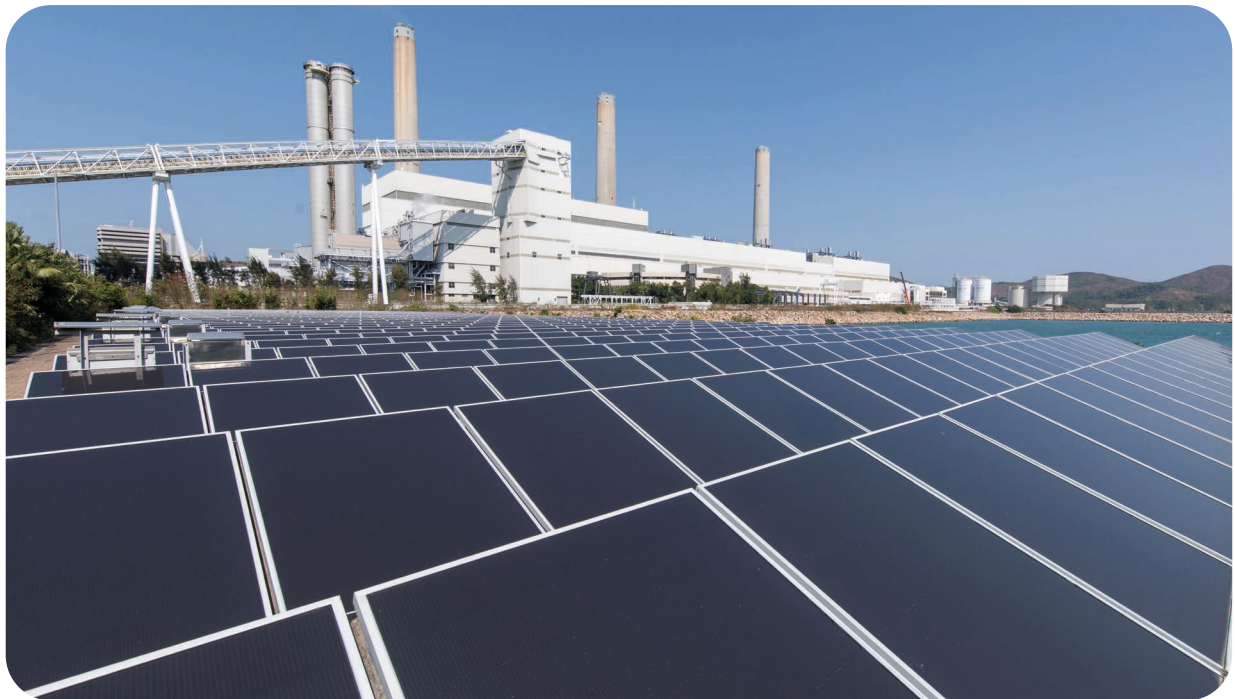
Solar panel station at Lamma Power Station, HK Electric
