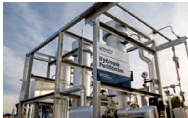
Australian Gas Infrastructure Group 的 Hydrogen Park South Australia
