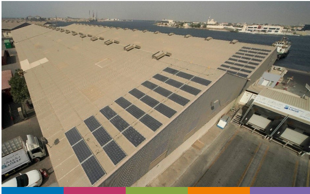
Solar Panels installed on the roof of warehouse in Hutchison Ports Ajman in UAE.
