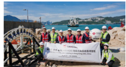
South East Asia-Hainan-Hong Kong (SEA-H2X) Submarine Cable successfully landed at China Unicom Hong Kong Tseung Kwan O L2 Cable Landing Station
