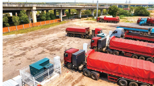
● New energy heavy-duty truck charging station in Nanchang City
