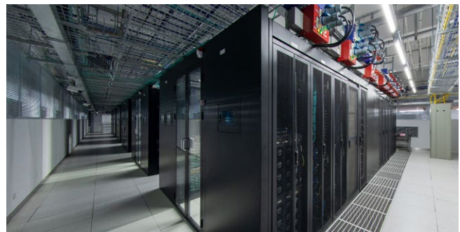
Domestically developed liquid-cooling intelligent computing cluster facility building with ten-thousand GPUs in one single pool in the Intelligent Computing Valley in Shanghai Lingang
