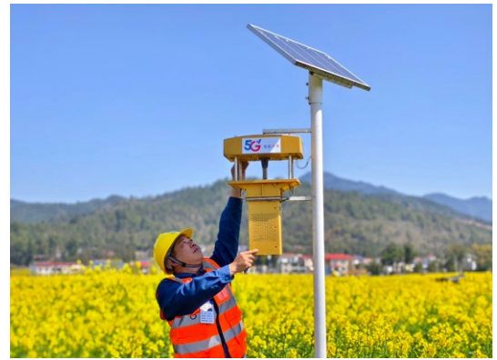
Workers debug 5G intelligent monitoring equipment
