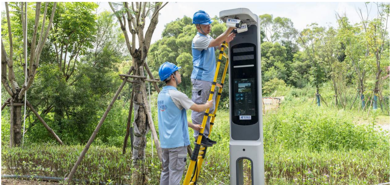
Technicians were debugging 360° AI signposts
