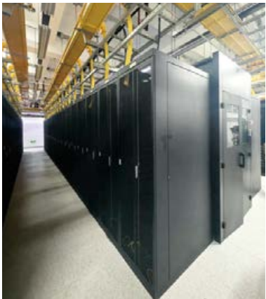
● High-performance Computing Power Center Construction Project for a Provincial Meteorological Bureau
