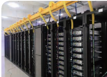
Digital Government Big Data Dedicated Cloud Machine Room Project
