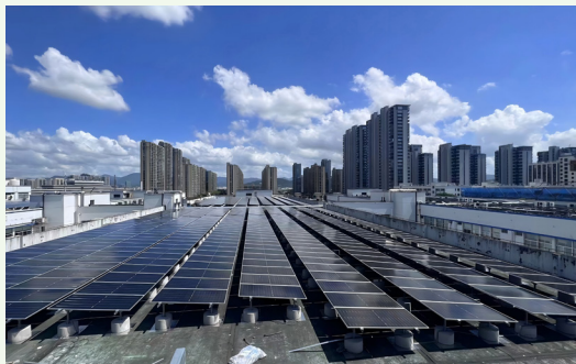
Supplier Rooftop Photovoltaic Project
