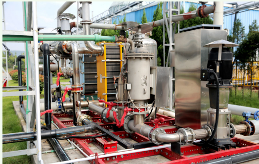
Supplier Waste Heat Recovery Project
