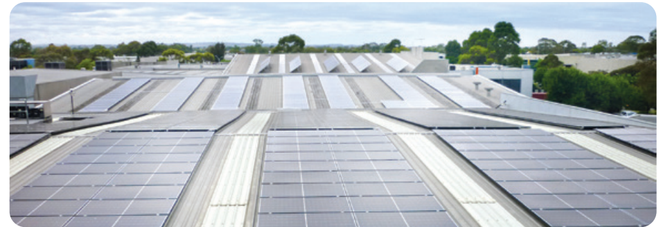
Solar panels implemented in Keysborough Site
