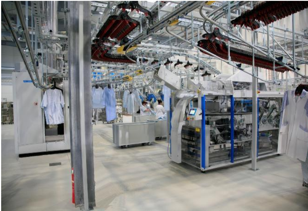
Supply and Installation of Laundry Service System for Garment Sorting and Finishing, Shum Wan Laundry
