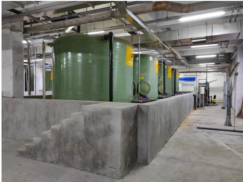
Wastewater Treatment Plant, Qingdao
