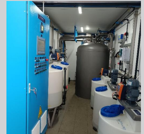
Tsuen Wan Water Treatment Works Ceramic Membrane Pilot Test
