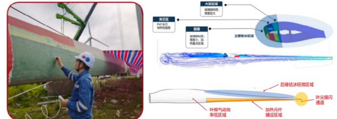
CP Hua Chuang Wind Turbine Blade Anti-Icing Coating Technology Application Site (Left) and Technical Schematic (Right)
